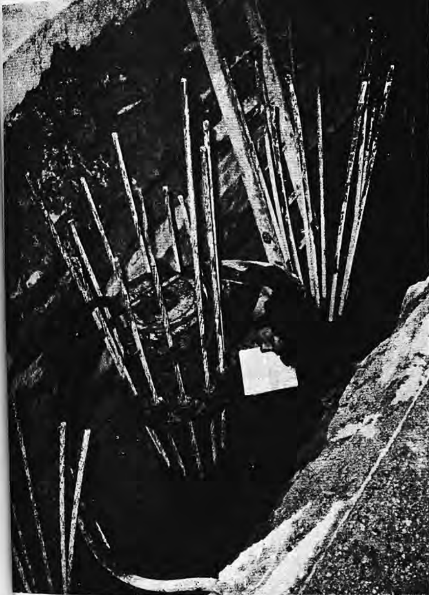
Fig. 8. An operator recording the tendon extension of a 2 000kN anchor during the course of multistrand stressing
