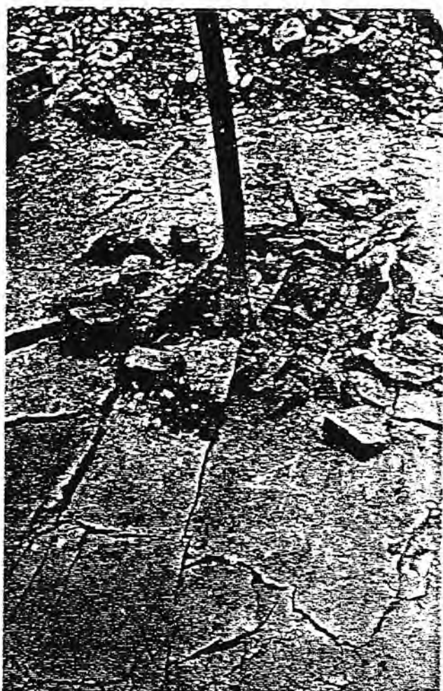
Fig. 2. — Failure volume induced at anchor 4, showing the control of the dominant NW-SE joints.
