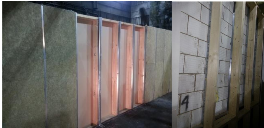
Figure 7.7. Sections prepared for inserting other insulation (a) before building up the aircrete wall - view from inside the compartment, and (b) after building the aircrete wall – view from outside
