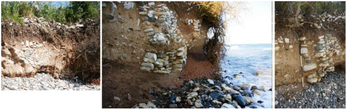
Figure 5. Wall in Building 1 gradually deteriorating between June 2010, June 2011 and January 2012 (personal photography).
