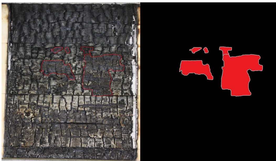
Figure 6.15: Back wall of experiment \beta -3 after deconstruction, showing manually identified delaminated areas (left) and MATLAB-produced monochrome image (right).
