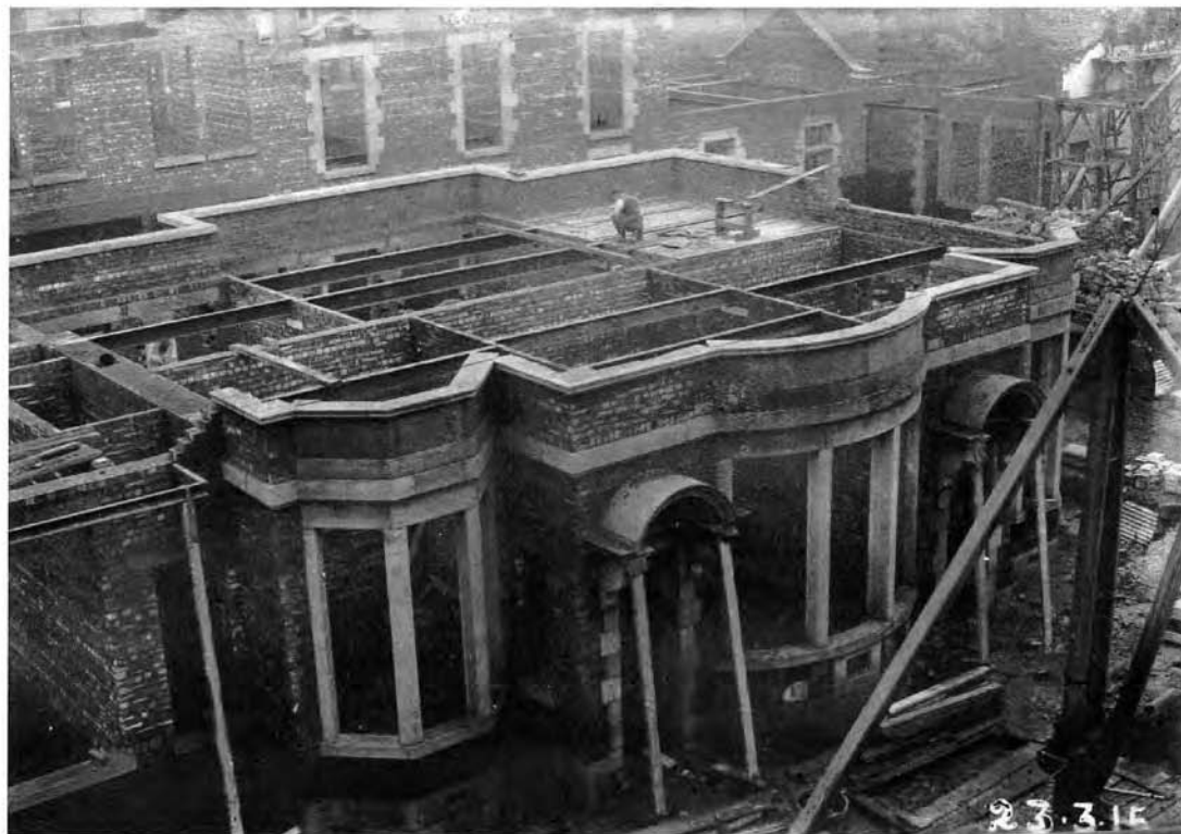
Fig. 9. The Construction of the Clinical Block Showing the Ground Floor of the Consulting Room and Pharmacy Block Completed. A Workman is Preparing the Dog Run and Loose Boxes etc in the Background [Dick Archive]
