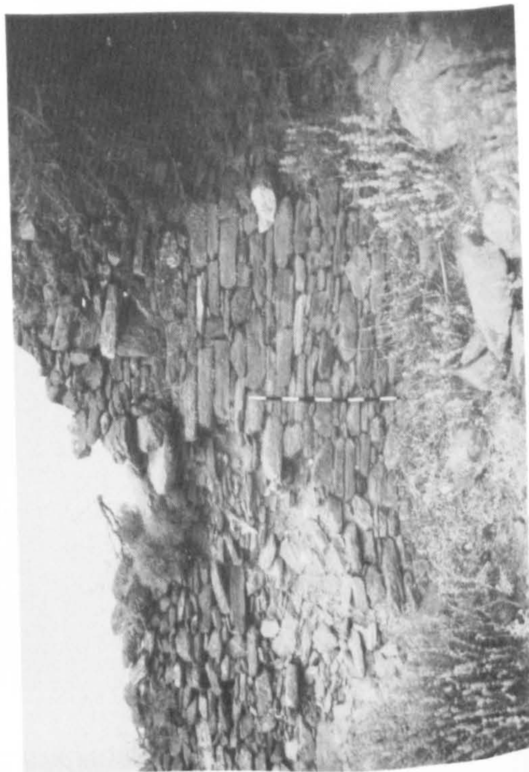
(d) AYIA MARINA: view from the N. (a) schist slabs; (b) low retaining wall.
