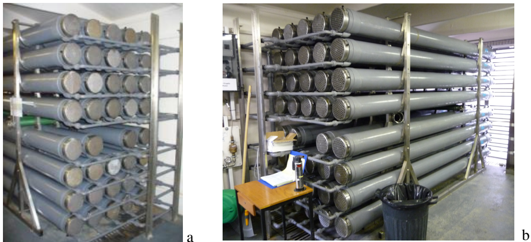
Figure A-1.1 Pictures of Plant A installed in a remote north island
