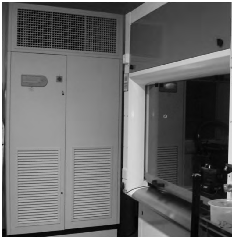
Figure 3-1. Environmental Control Unit
