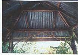
The views of the entrance porch and details of its roof structure
