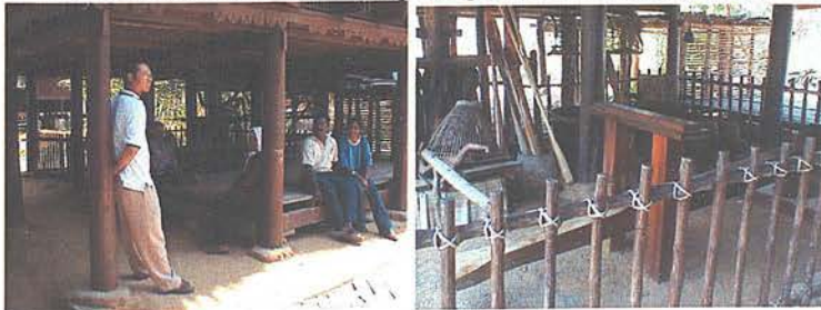
A view of the space underneath the elevated floors and how it has been used as a resting place and storage space for equipments.
