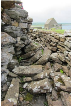
Figure 127 (left) Gallery void south of the high wall cell with slabs fallen from the RHS now pinned under the outward bulge of the inner wallface.
