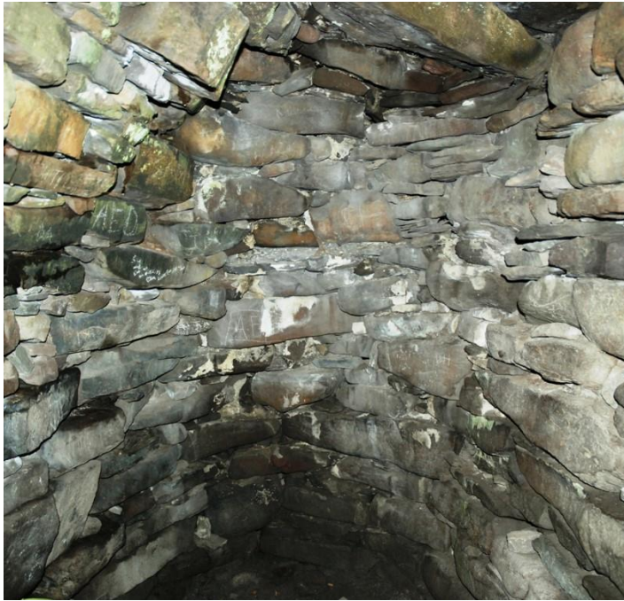
Figure 81 (left) Cell A. The wall on the right is probably an original gallery wall. The LHS wall is topped with what has been called corbelling. However, this masonry has simply fallen inwards and wedged in place now apparently stabilised with mortar. It is not a drystone built feature and cannot have been one, given the sloping joint planes.
