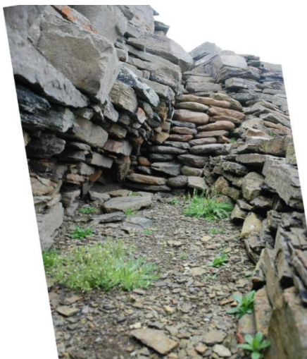
Figure 117 View along gallery floor towards the south end of the outer wall breach
