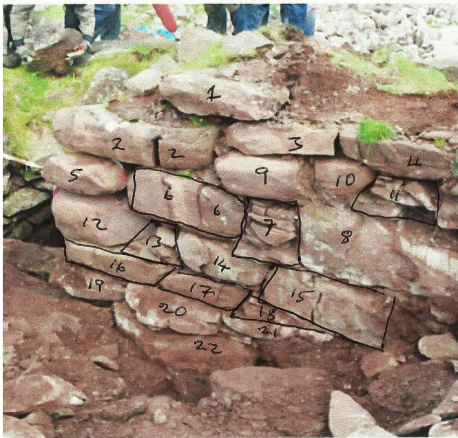
Figure 173 A crack swarm in masonry right of the stacked void over the entrance passage at Clachtoll. Stones 2, 9/10, 11, 6, 7, 14, 15 and 21 were broken when revealed. In the wall core virtually every stone was cracked or broken.
