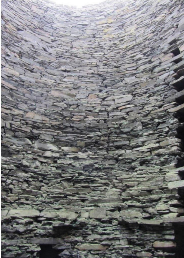
Figure 74 Major structural cracks are clearly visible in the inner wallface. Note apparent displacement of the LHS wall of the second void in comparison with the lowest.
