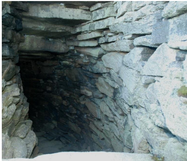
Figure 146 A view down the composite stairway with the stepped risers visible at the top of the image.
