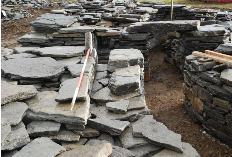
Figure 50 The barhole and slot under construction in a 1:1 model of the Clachtoll broch entrance area. Given the small cross sectional width and height of the barhole and the narrowness of the entrance, failure to insert the bar at this stage would preclude its insertion later.
