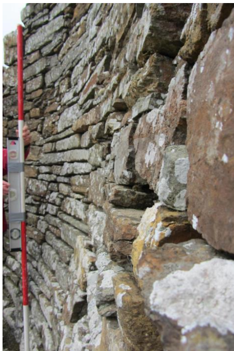
Figure 128 (left): The profile of the Inner Wallface adjacent to and below the 1 o'clock high cell. The ranging rod is vertical.
