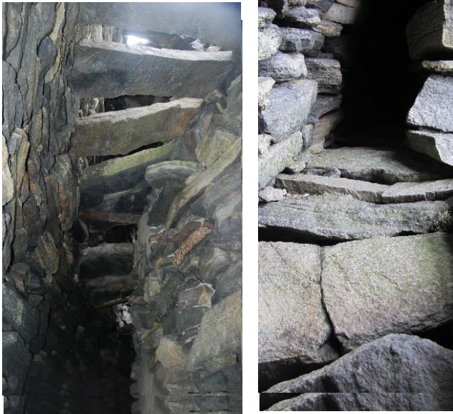
Figure 137 a (far left) The broken and displaced lintels of the third level. Their displacement and the buckling visible in 137 b (left) confirms that the intramural void is now narrower than it originally was. These indications suggest that the outer wall has also slipped downwards and inwards and moved slightly, anti-clockwise relative to the inner wall.
