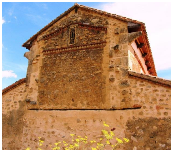
Figure 18 Evidence for earlier wall and roof lines surviving in the external face of the east elevation of the church at San Miguel de la Escalada.
