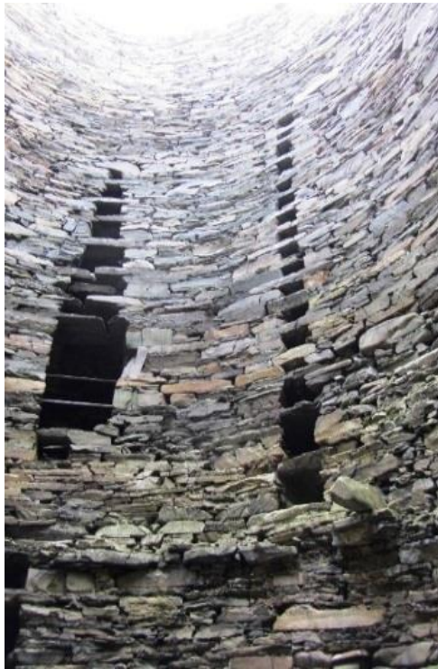
Figure 71 (above) Stacked voids above the stairway entrance.
