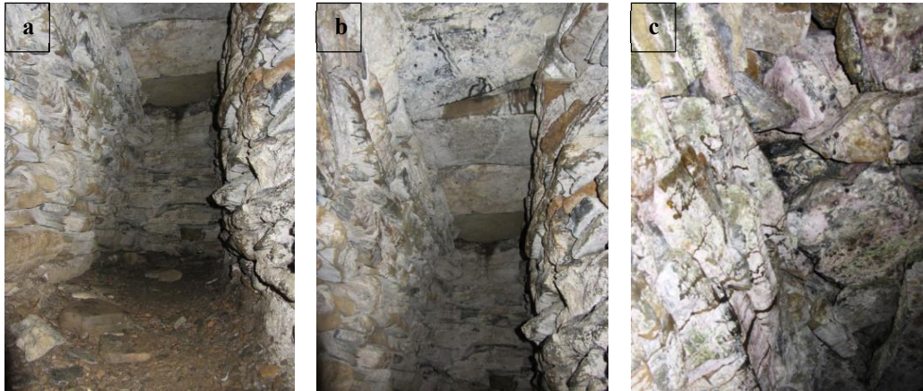
Figure 129 a, b and c The anticlockwise end of the LHS ground gallery at its blocking at 9 o'clock (a). Here its roof lintels are intact (b) but closer to the guardcell, the roofing lintels have failed and chaotic structural debris has bridged the gap (c)
