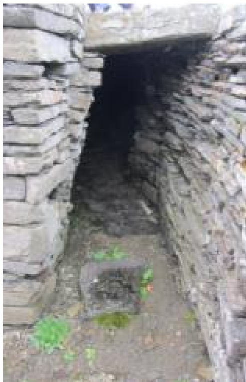
Figure 93 (left) Entrance to the intermediate gallery, now inclined to the outside of the broch by an average of approximately 15 degrees.
