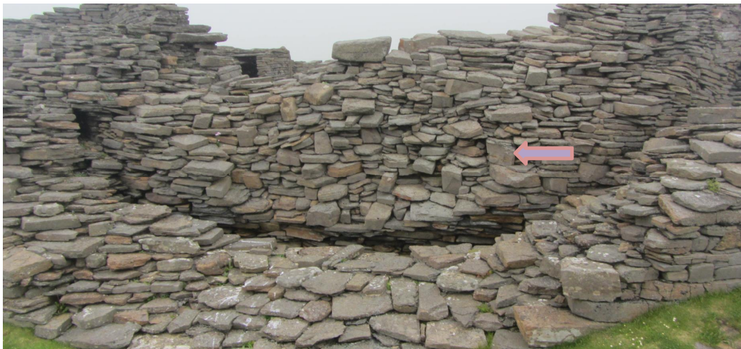
Figure 114 The breach of the south wall. The apparently vertically set stones, like the one indicated, have their horizontal bedding-planes set in the horizontal building plane and their 30o/60o cleavage-planes in the vertical, the better to resist compressive forces.
