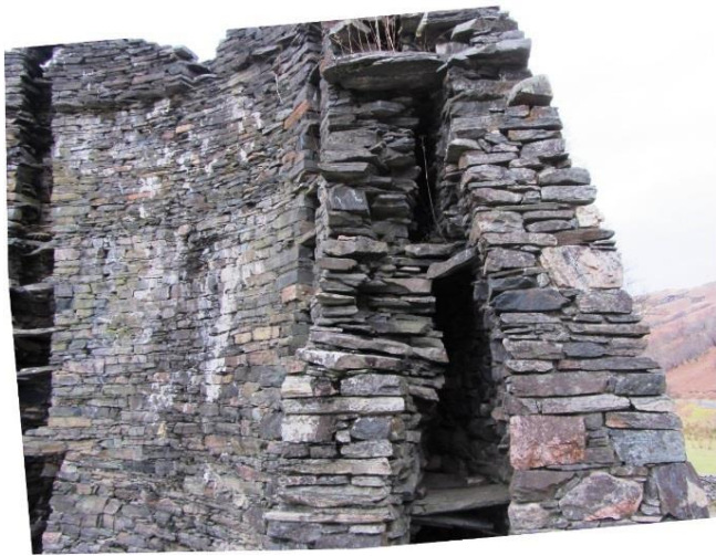
Figure 155 A localised defect in the inner wall on the northern edge of the high masonry at Dun Telve. The squared return at the foot of the image marks the line of the edge of a stacked void (subsequently conserved), beyond which the wall fabric bulges inward, breaking and displacing lintels, above and below. The neatly squared return on the lower outer wall is wholly an artefact of conservation.
