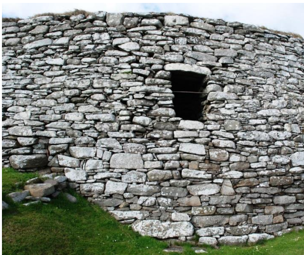
Figure 82 (left) The tertiary entrance at Clickhimin. Rispain joints isolate the block of masonry immediately below the entrance, which may have extended down to the level of the masonry abutting the broch left of the ope; but note earlier repairs below this level.
