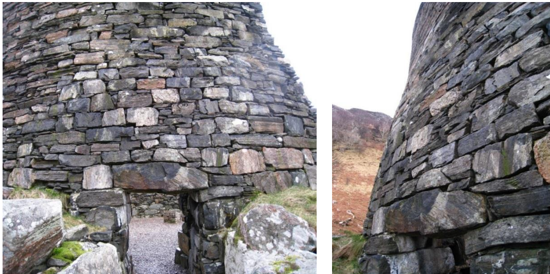
Figure 152 a & b The bulge of restored masonry over the entrance at Dun Telve. In the frontal image the rebuilt occupies the greater part of the image area but differences are obvious between the rebuild, mainly of large squarish blocks of stone, and the original, mainly of the relatively thin flat slabs visible in the upper left and right corners of the image. Image b (right) shows the bossing of the inserted masonry, out of line with the smooth conical surface of the outer wallface behind it, as viewed here.
