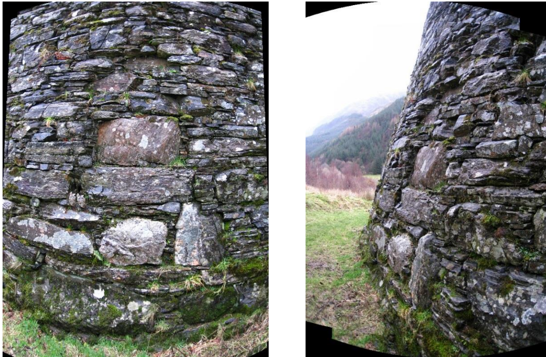
Figure 171 a & b. An infilled breach in the outer wall outwith the stair cell entrance. Both images are panoramas and parallax distortion is obvious but the inseting of the wall is clear and is real.
