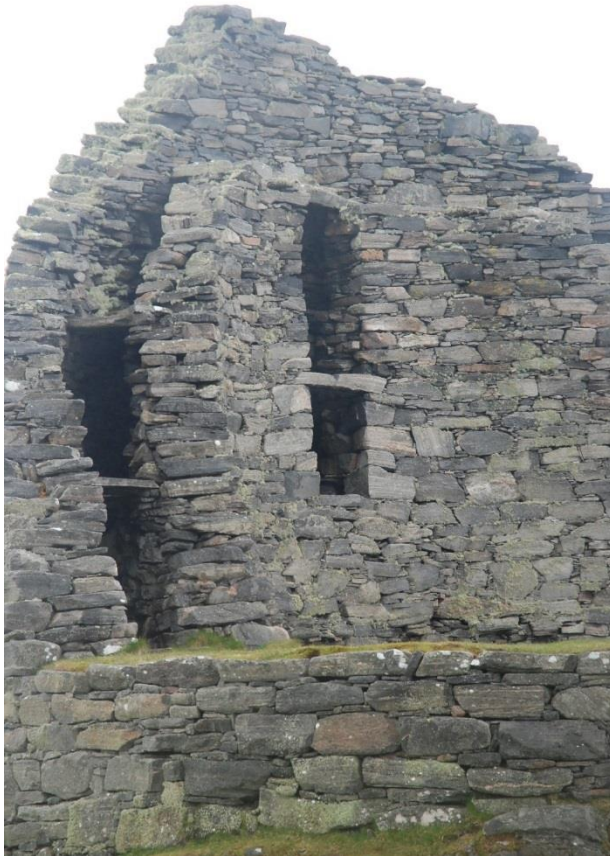
Figure 138 The edges of the inner wall curve inwards to produce a conch-like form, a consequence of the failure of its surrounding wall, which pulled the remaining edges with it as it fell.
