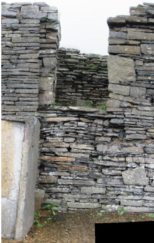
Figure 92 The masonry directly under the ope is badly disarranged and it is likely that it blocks a door ope that gave access to a ground floor gallery or a ground floor stairway, possibilities that can only be tested by excavation.
