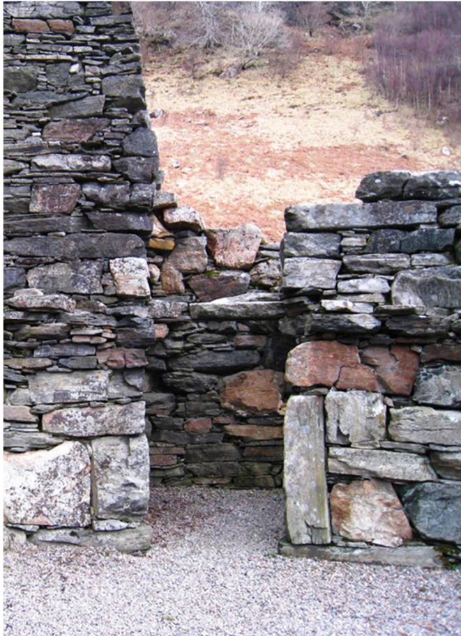
Figure 164 The first four courses above the left hand edge of the stair entrance ope in the inner wall, on the basis of the 1916 survey, forms part of a lost stacked void return. The right hand edge seems to confirm this identification but may have been rebuilt.
