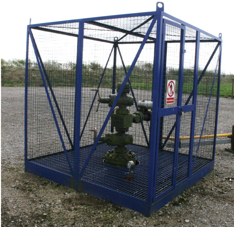
Figure 5-6 – Photograph of the steel cage around the Elswick-1 wellhead. The wellhead is connected by a pipeline (yellow, in the background) to an electrical generator.
