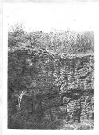
Lateritic concretions in borrow-pits at Daura. Note the pencil and the camera case for comparitive sizes.
