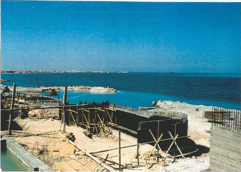
Figure 6.27: Heavy constructions on the already land filled site, the new extension of 'Felfela' restaurant. Note bay extending to the reef edge. (8/1993)
