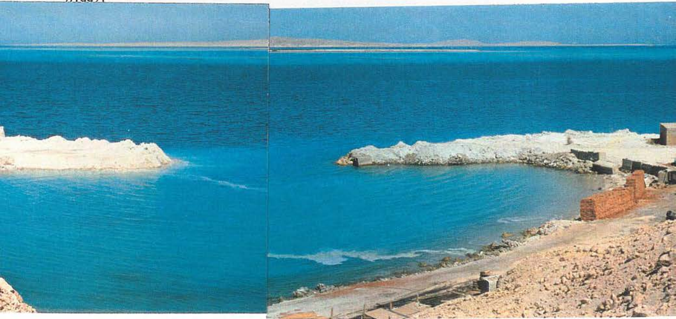
Figure 6.26: August 1993, concrete blocks and red bricks forming land filling to create the man-made bay at Felfela site.
