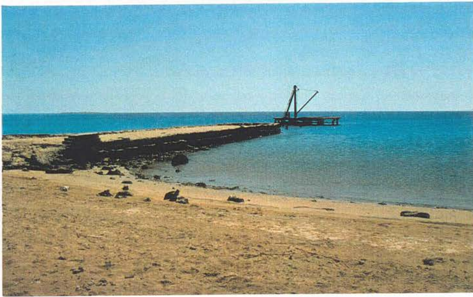
Figure 6.83: A derelict landing pier on one of Hurghada's off-shore islands, built to provide access to fishermen. (7/1992)
