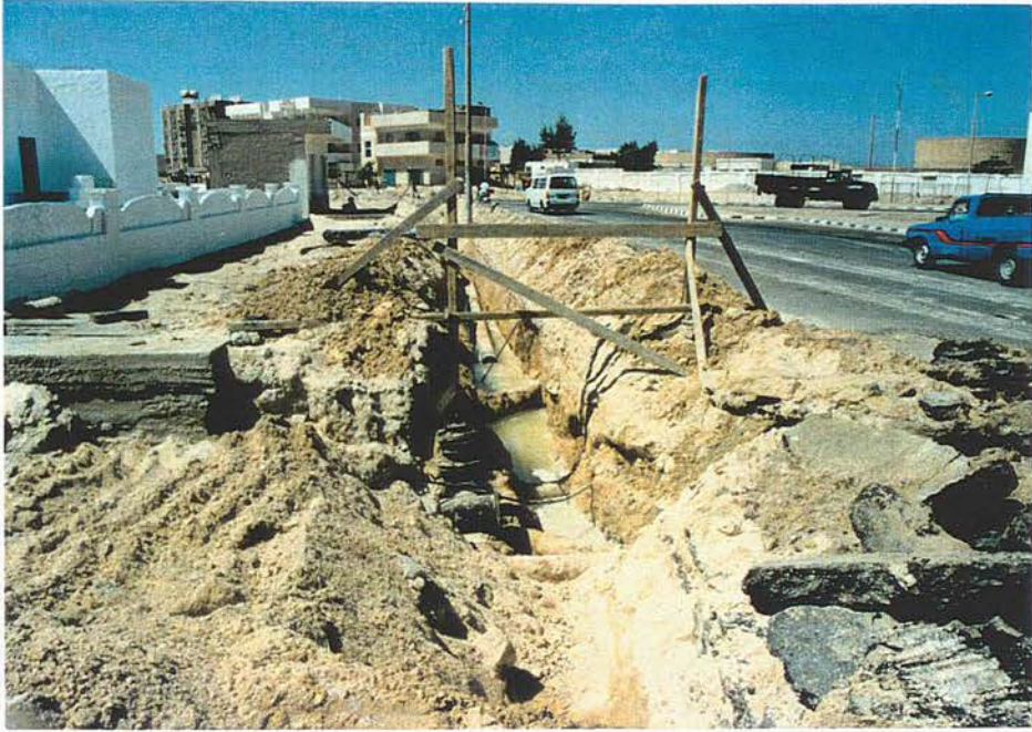
Figure 6.86: Work at Hurghada on the sewage system under construction in August 1993, still catching up with development.
