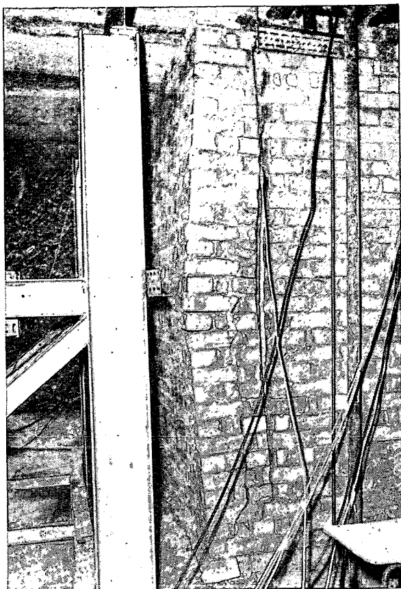
Fig. 6. Typical failure of wall with return
