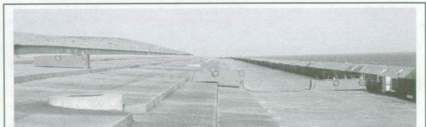
Figure 4. Overtopping tanks at Samphire Hoe.
