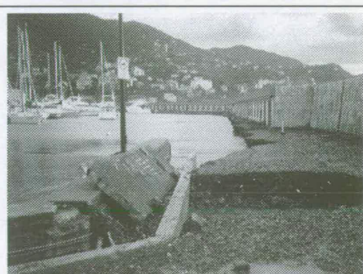
Figure 14 Overtopping damage at Rapallo marina
