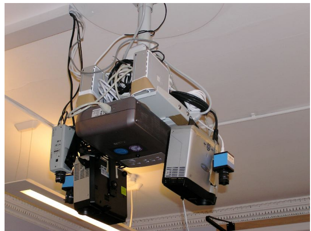
Fig. 1. The two projection systems (Mac mini, projector and camera) mounted above the table next to the projector for the projection screen in the old instrumented meeting room. The grey camera is part of the equipment used for meeting recordings.
