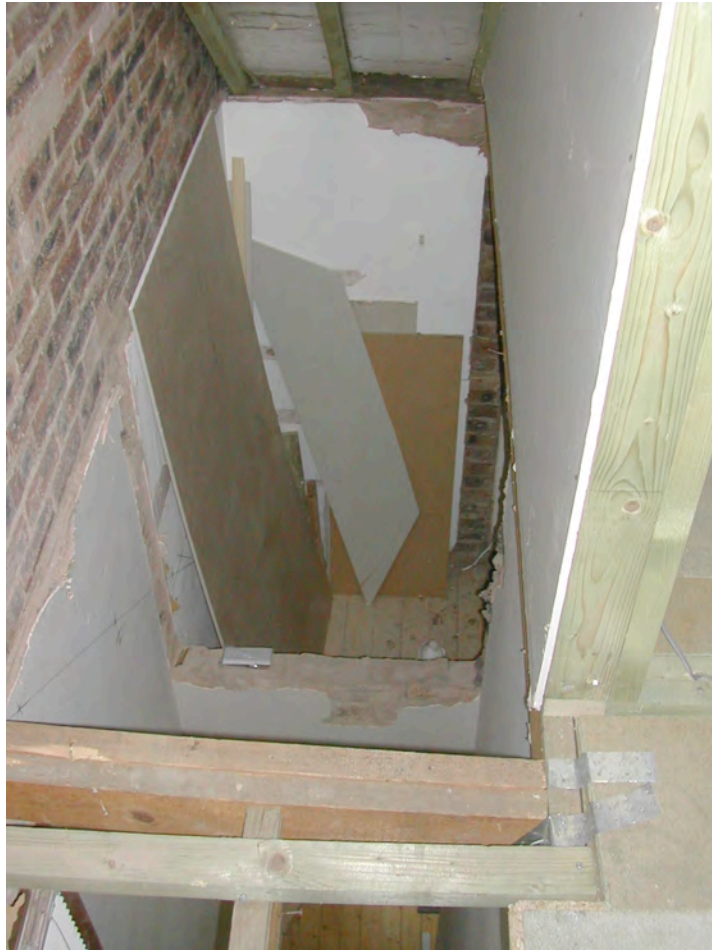
Figure 6.4 Staircase opening, as it remained until the architect intervened
