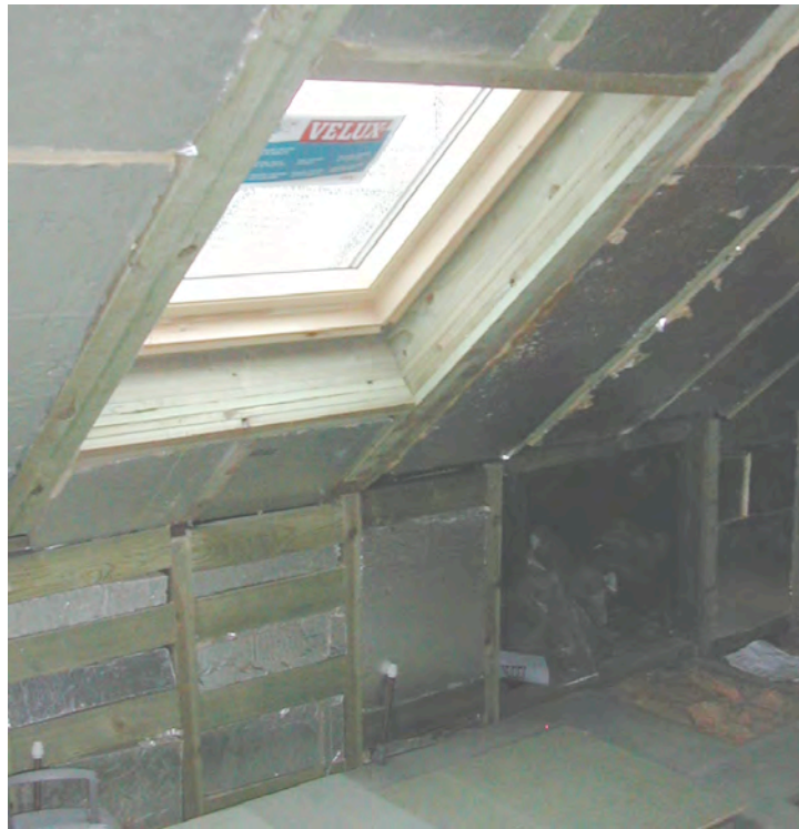
Figure 6.3 Fire escape window in-situ
