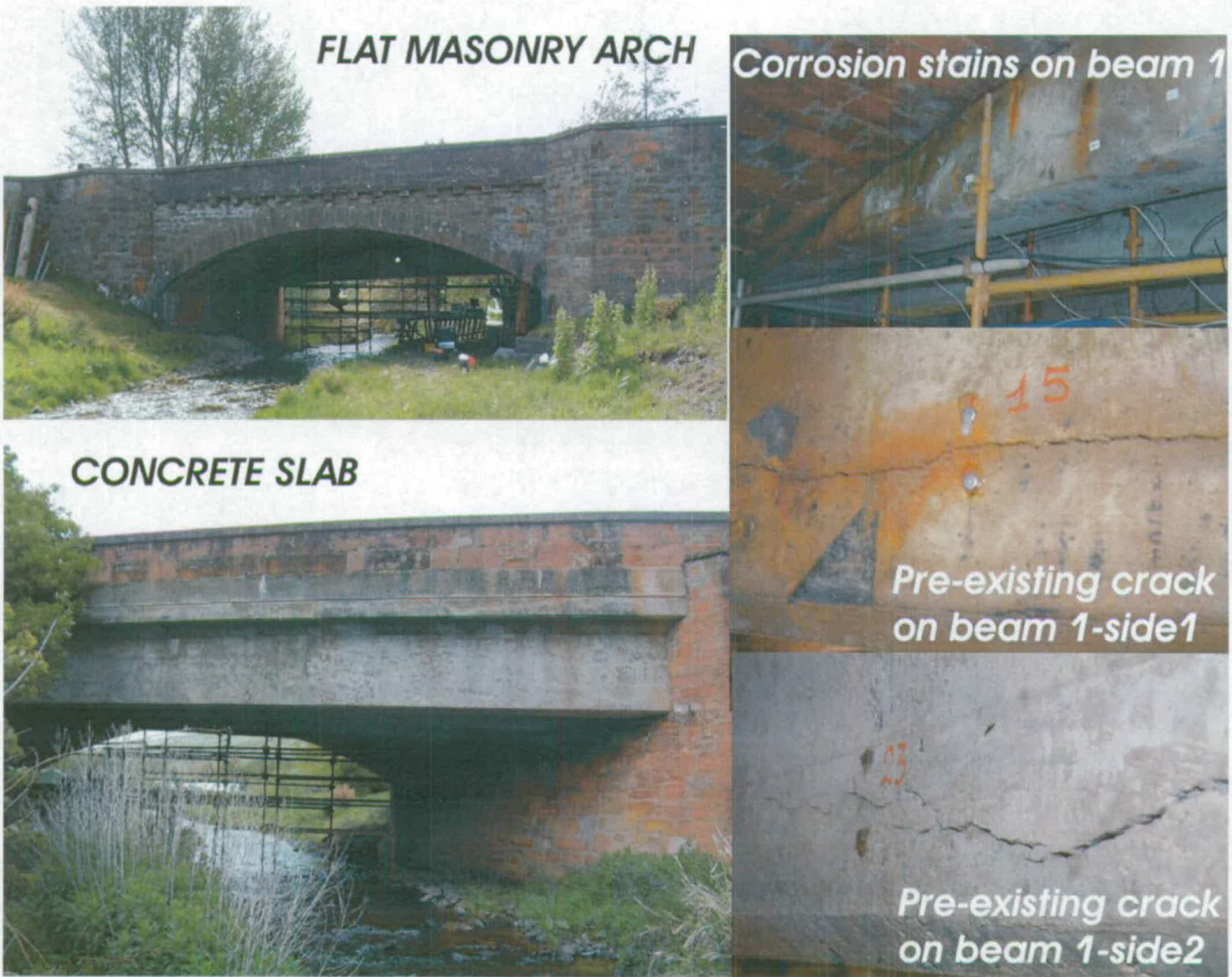
Figure 8.1: Boghall bridge: masonry and concrete side; pre-existing cracks.
