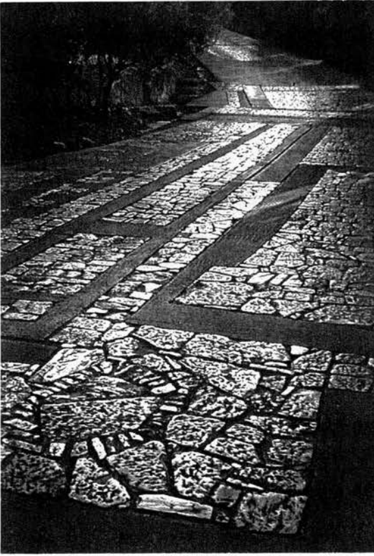
Figure 8.27. Reinforcement of the pavement of the road leading up the Hill of Philopappus with concrete where it was intended to be used by vehicles.
