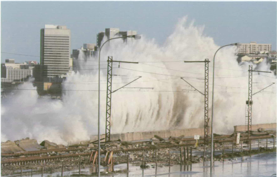
Figure 2.2 Overtopping damage to railway infrastructure in Port Elizabeth, South Africa
