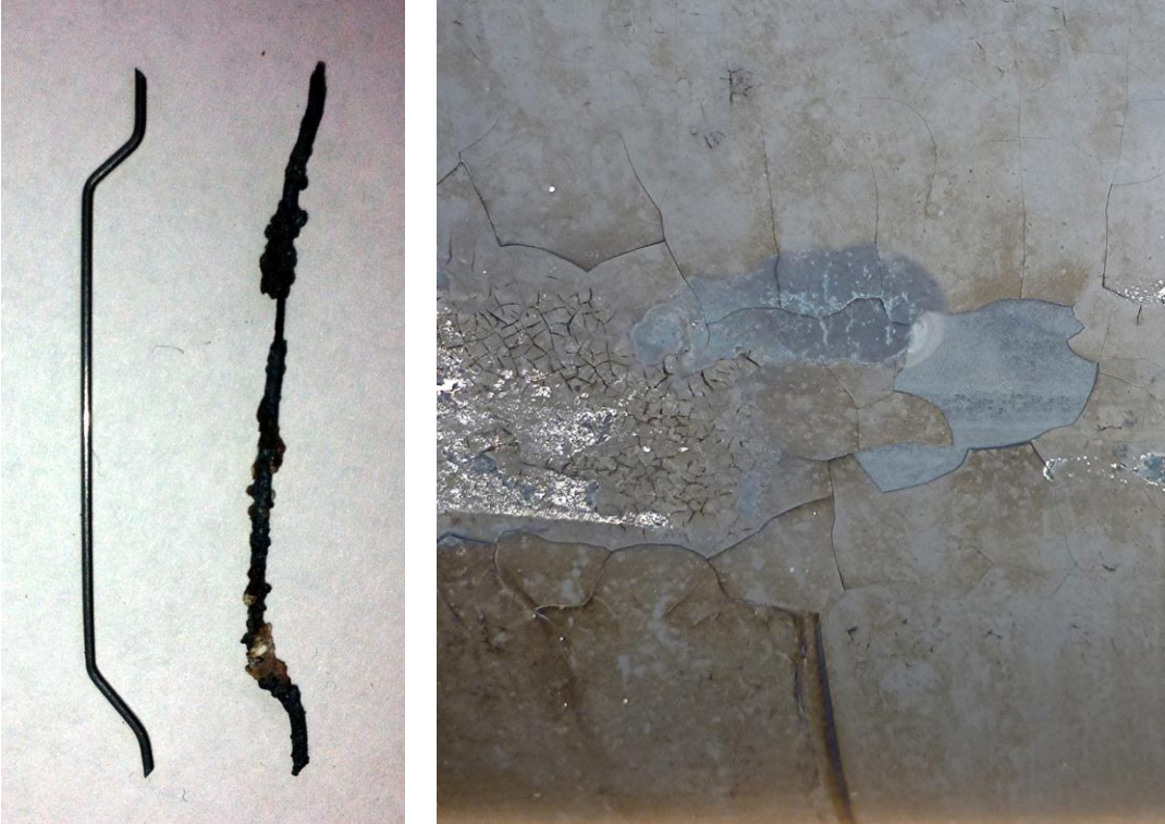
Figure 7-1: (a) Comparison of steel fibres pre- and post- thermal insult; and (b) surface slag on exterior steel on unprotected CFS columns
