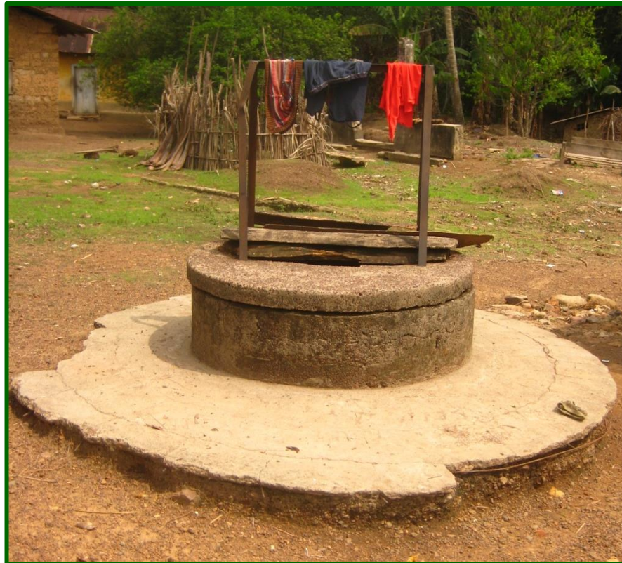
Figure 32: Severe erosion on older well type caused by lack of drainage - Patifu
