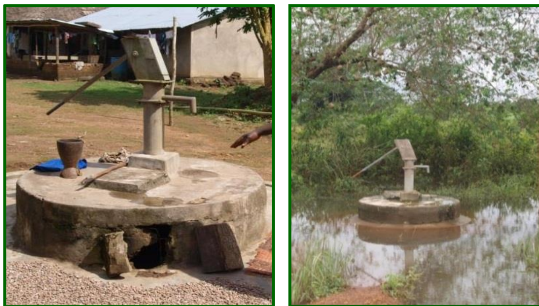
Figure 45: Examples showing Grade A hand-pump well failures
