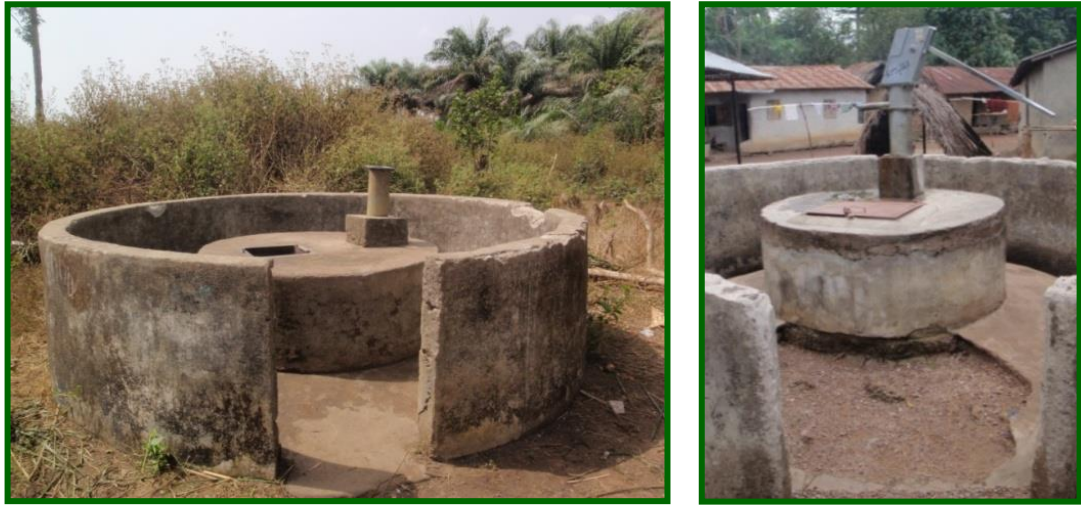
Figure 46: Examples showing Grade B hand-pump well failures
