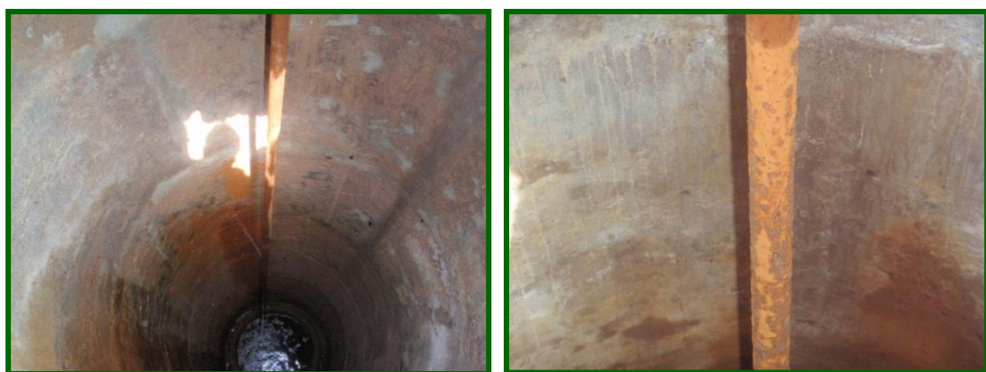
Figure 35: Example of Grade C failing - Mabang
