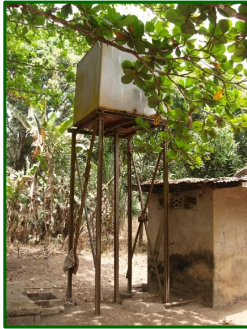
Figure 21: Example of a pre-Mano River war piped system - Kumrabai Station
