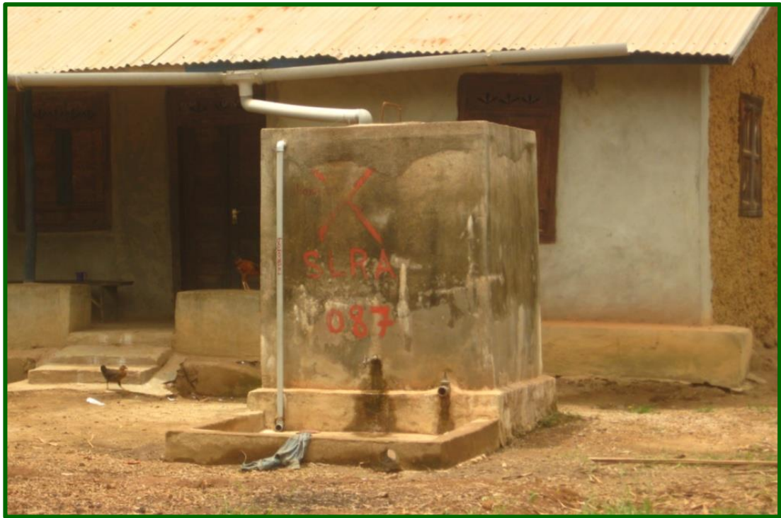
Figure 85: Example of a permanent rainwater harvesting systems - Bongay
