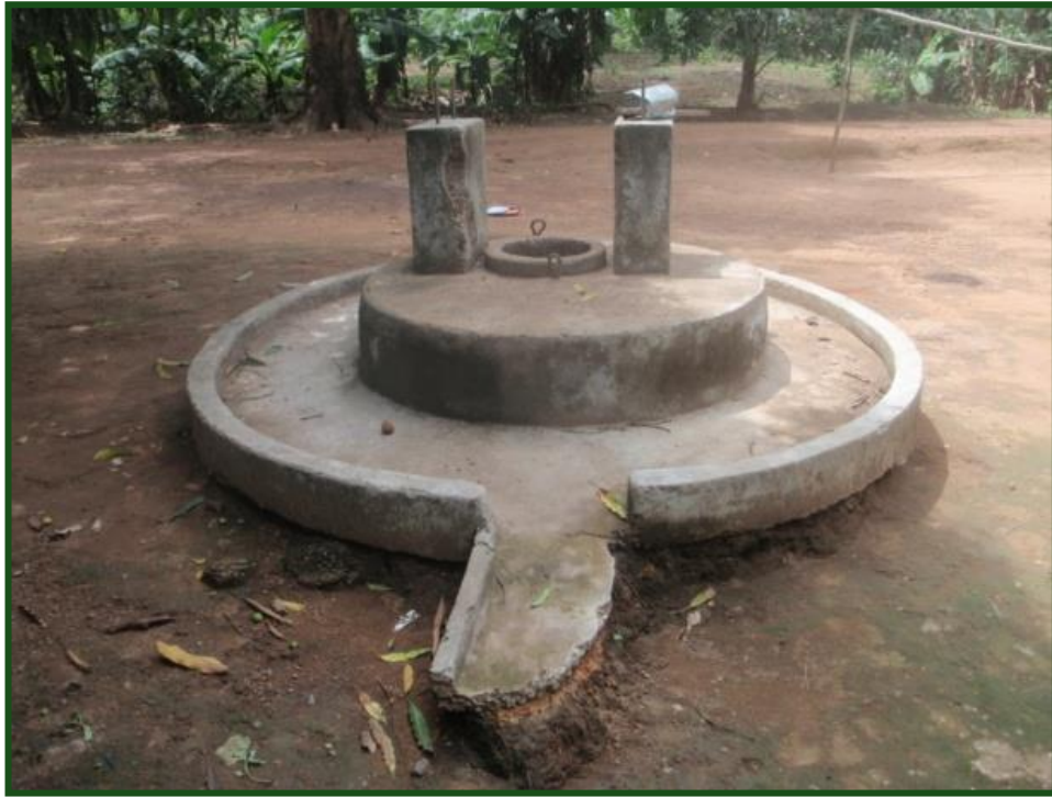
Figure 39: Multiple Grade B and C failings on the one source Mabum Station
