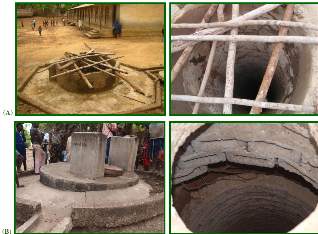
Figure 33: Example of Grade A failing (A) Patifu (B) Masokoh
