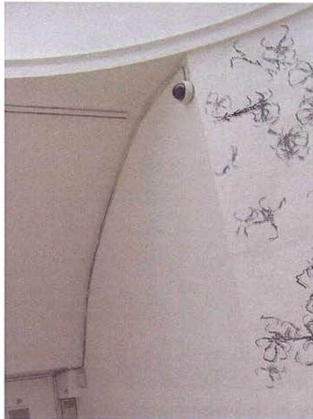
Figs. 73 & 74 Round Room details (skirting board on top, electric wiring on bottom) BEFORE being painted white
