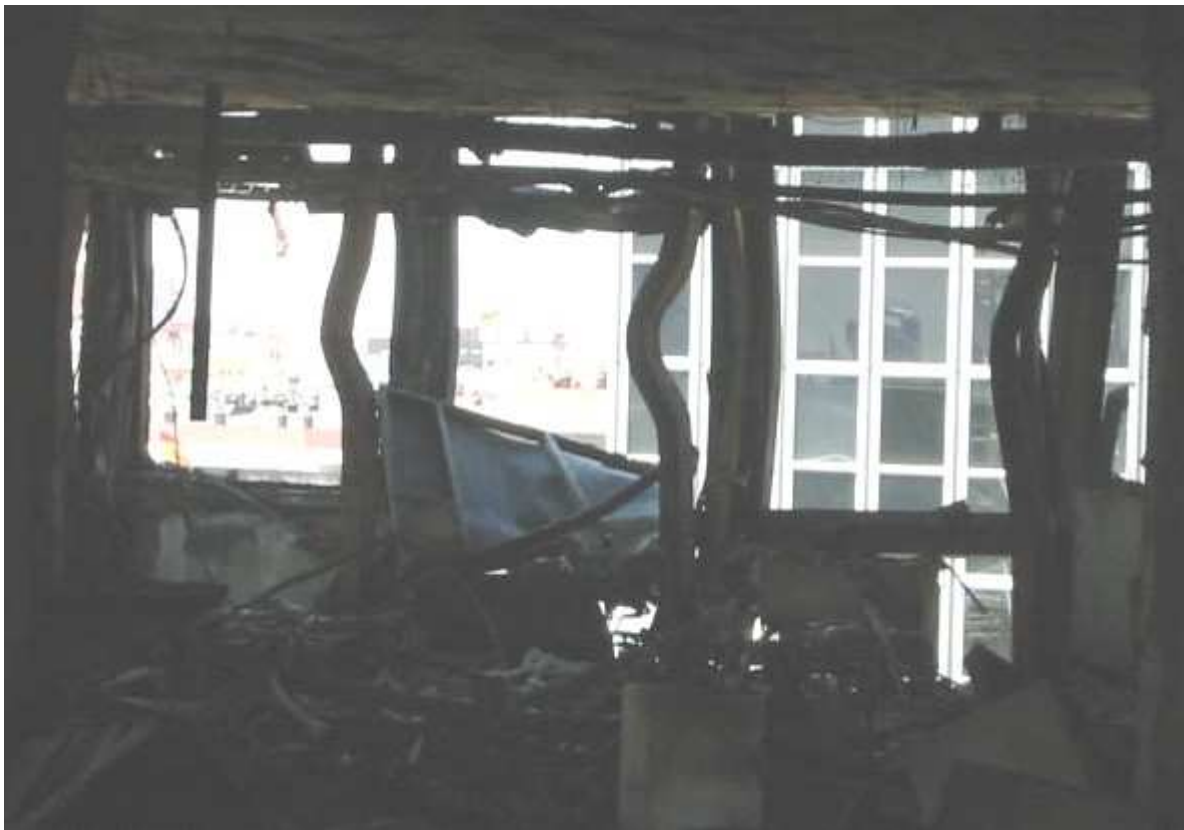
Figure 2 – Buckled steel columns on 9 th floor, photograph from The Concrete Centre
