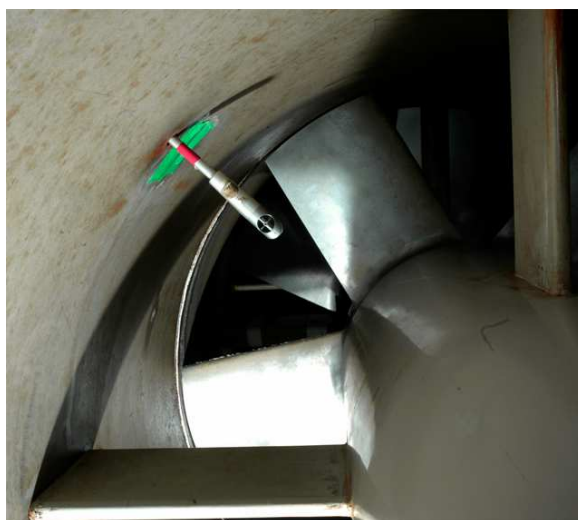
Figure 74: Vane anemometer in turbine duct upstream of turbine blades
