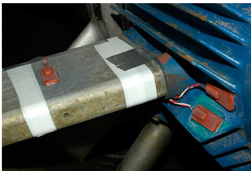
Figure 73: Mounted surface temperature measurement sensors
