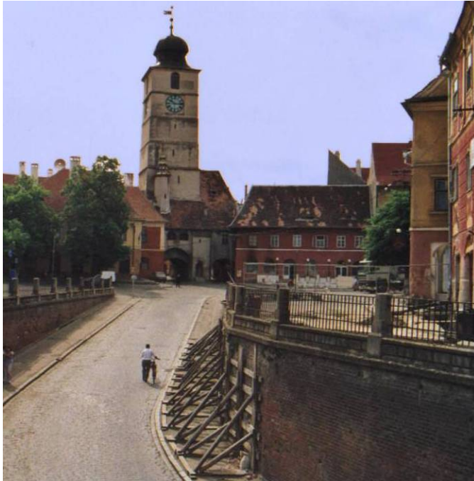
Figure 111. Sibiu, Lies' Bridge retaining wall propped with wooden beams to reduce bulging and avoid collapse due to land sliding
