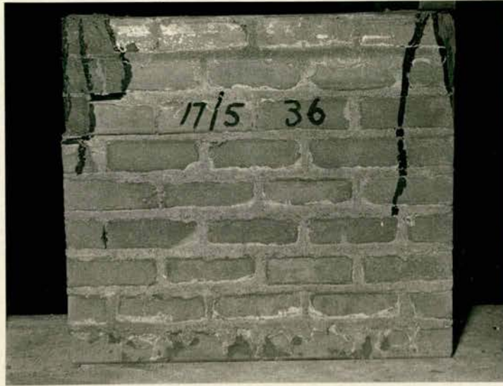
1/3rd. Scale Brick Wall - End Bearing Plate - Failures by Local Spalling, Crushing and Vertical Cracking.
