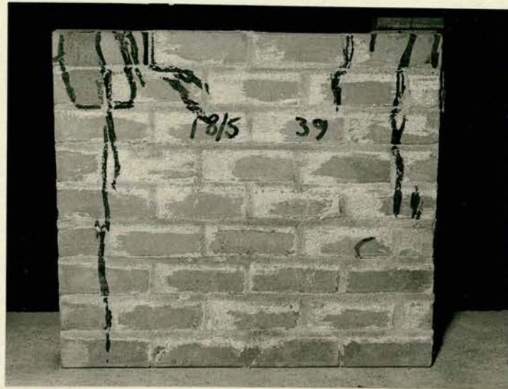
1/3rd. Scale Brick Wall - End Bearing Plate - Failures by Vertical Cracking and Spalling. Plate 6-3
