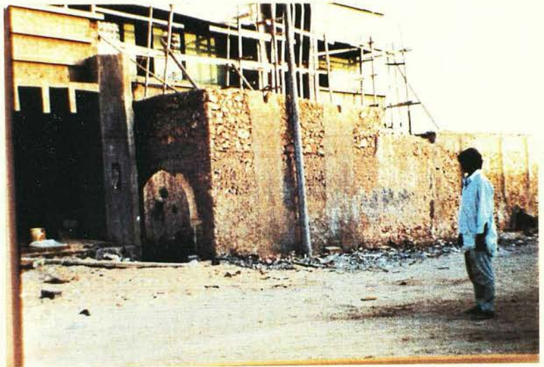
Fig 6.66 The old wall of a traditional house is retained until the new house is complete. The author monitored this area and remained until the wall was demolished (Fig 6.52).
