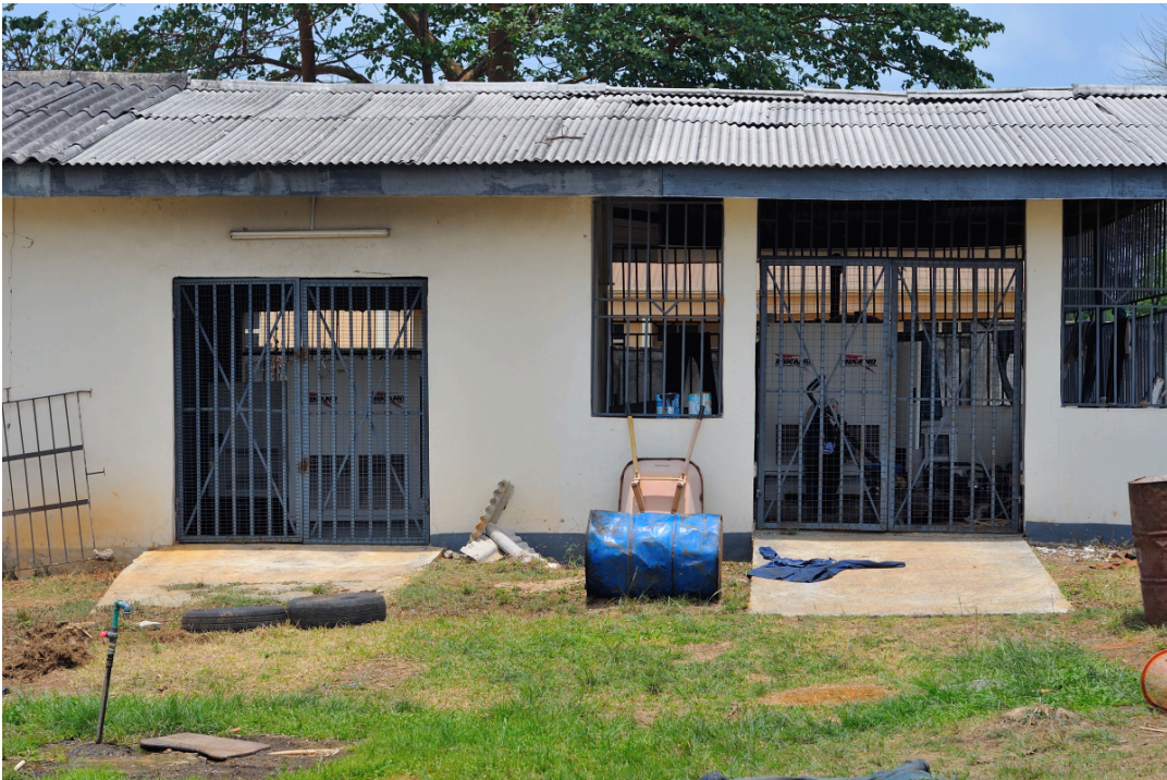
Figure 54 Large generators for power supply at RECTAS, OAU, Ile-Ife (Thorpe 2016).
