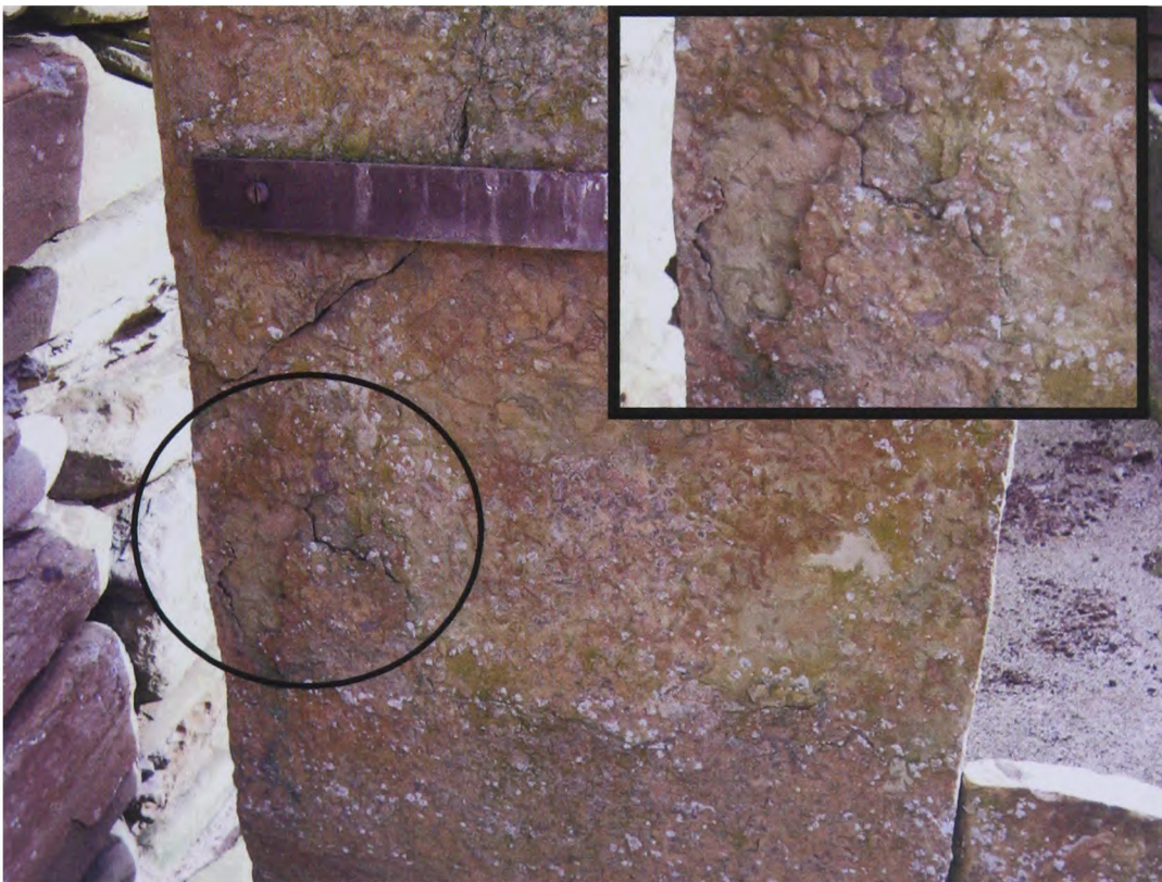
Figure 5.43: Cracking and damage on stones in House 1. Small corner image is a magnification of the circled area, which is estimated to be 20 mm wide. The scale of the stone 'furniture' is very similar to House 7.
