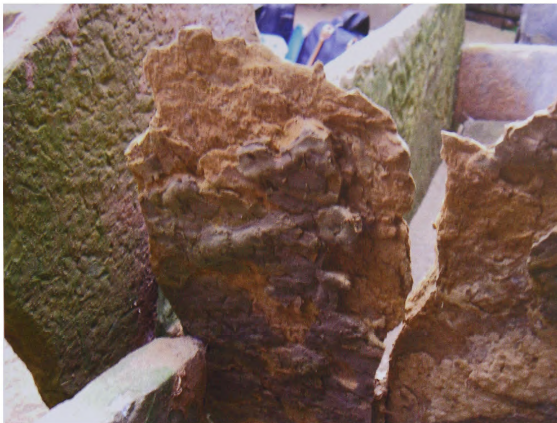
Figure 5.5: One of the worst areas of decay, showing the top of the slabs weathered to a thin sharp point. Photograph taken during the March (2004) visit. This is also the area where the data logger for the house is located. Stone slab in centre of image is approximately 71 cm tall, 24 cm wide and 2.5 cm thick tapering off towards the top. Area 3.
