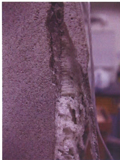
Figure 2.1: Cordova limestone exposed to routine sodium sulphate laboratory testing (samples are 5 x 5 x 25 cm). a) after 8 days there is no sign of efflorescence but the sample has begun to crack. b) after 47 days a layer of stone has separated from all over the surface. c) a closer view of the sample shows columnar salt crystals growing from the surface under the separated layer. Images and caption courtesy of G. W. Scherer, Princeton University, USA.
