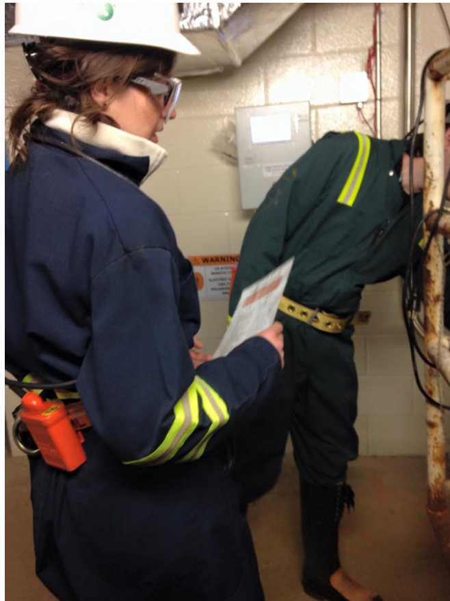
Figure 3.14 Davis Cavern (SURF): a colleague and I operating in one of the tunnels to refill the liquid nitrogen storage tanks.
