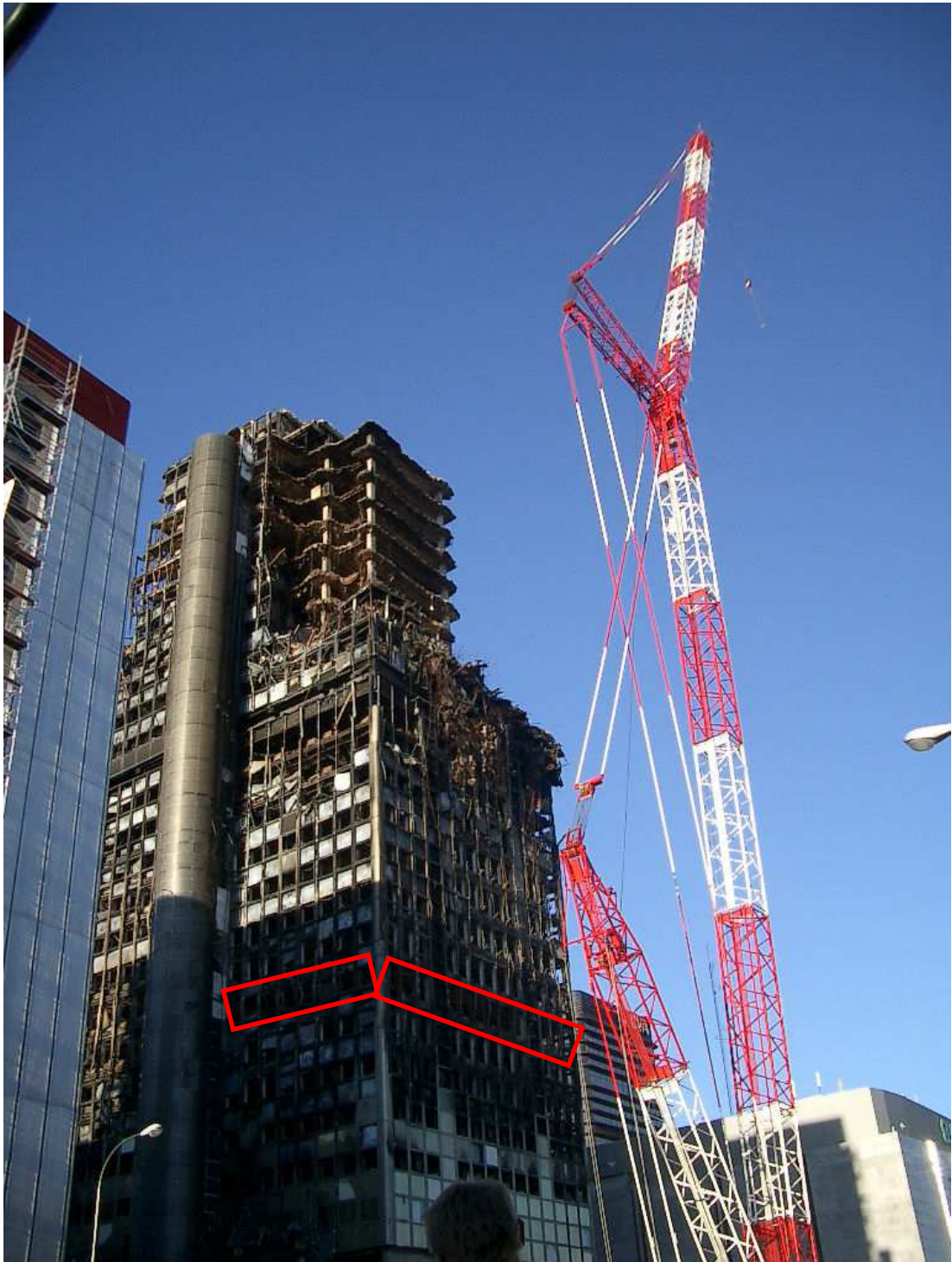
Figure 3.8 Post fire damage, 9 th Floor Highlighted (Daniel Alvear Portilla, Group GIDAI, University of Cantabria)
