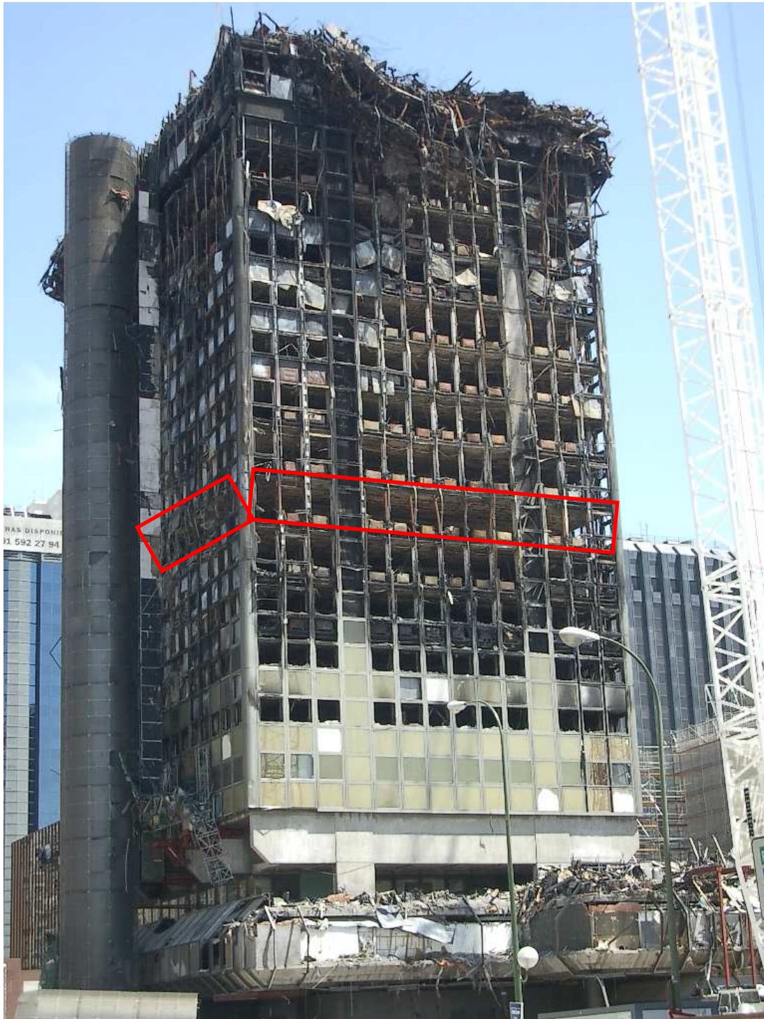
Figure 3.9 Post fire damage with demolition partially complete, 9 th Floor Highlighted (Daniel Alvear Portilla, Group GIDAI, University of Cantabria)
