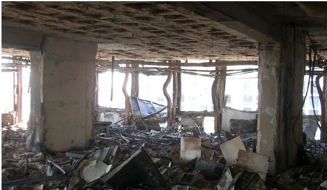
Figure 3.7 Post fire damage, Buckled Columns (Daniel Alvear Portilla, Group GIDAI, University of Cantabria)
