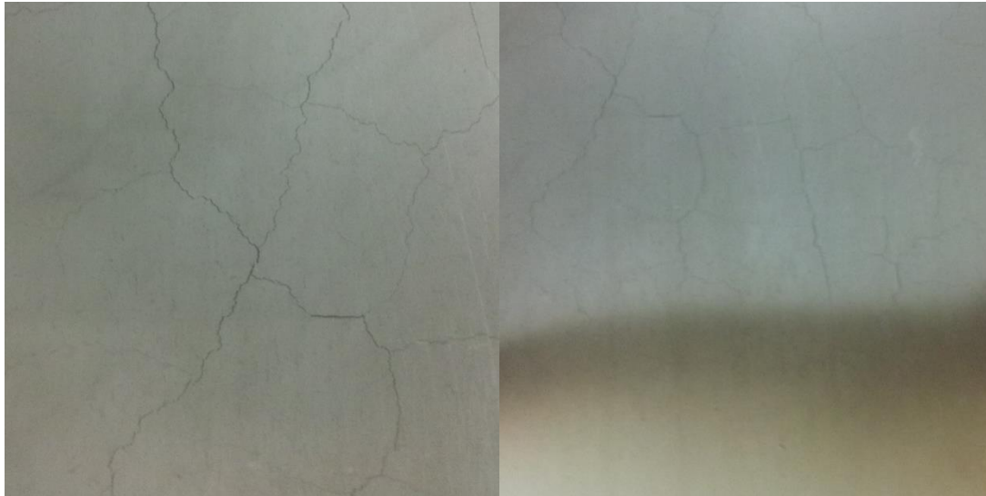
Figure 7.33 - Some crack patterns from the bottom section of the short wing, test 2 (a) general crack pattern across main burning area (b) cracking desists outside main area of burning.
