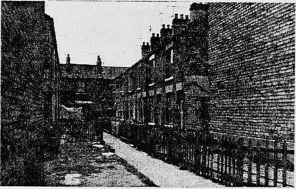
Unfit and socially unacceptable — highly decayed with dampness and structural faults.
