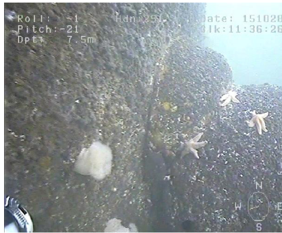
Figure 8.2: ROV Footage from Teesside Wind Farm showing marine growth on a monopile foundation [257].
