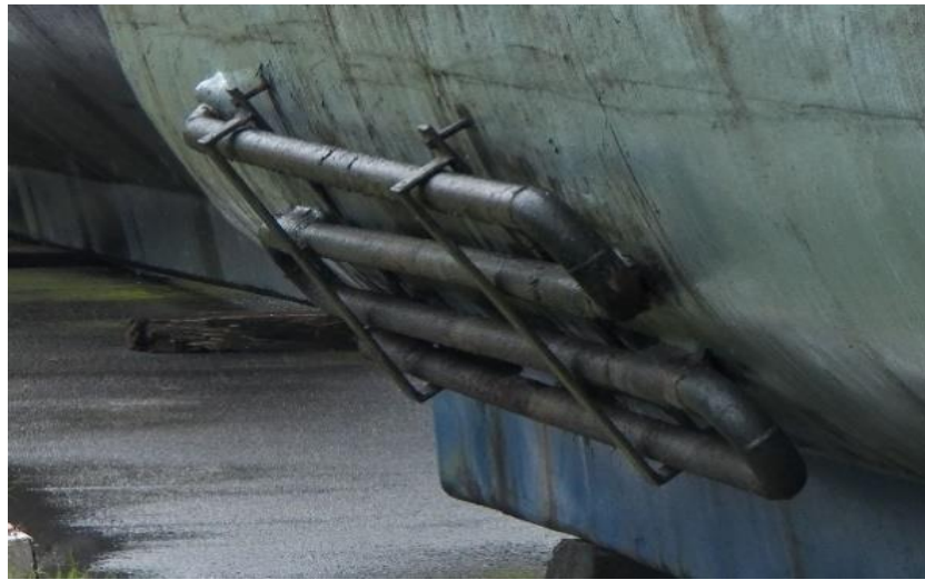
Figure 40. Heat exchangers. Source: Author.
