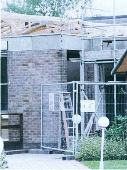
Image 4.2: Exploraway . This was where a female teacher, together with a male student who had a learning difficulty sat on the pathway near the construction fence. No seats were provided here.
