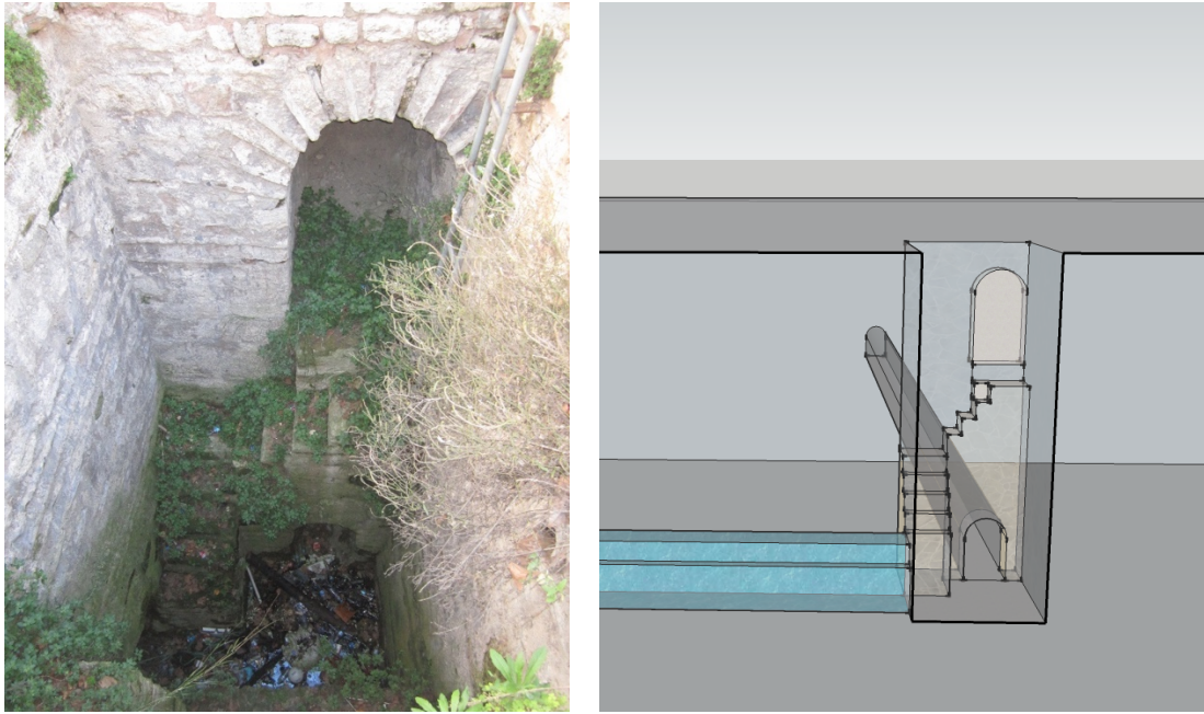
Figure 3.3: Structure to the north of the Aspar cistern. It may have been used to control water flowing from the cistern. Left – photo (K Ward). Right – sketch (F Ruggeri).
