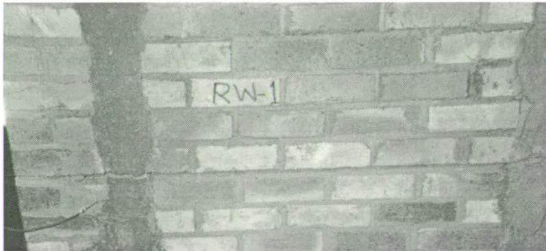
Fig 5.5 : RW1 after test (showing pocket side)
