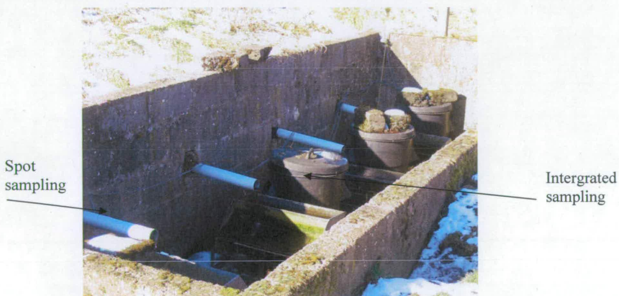
Figure 6: Drainage pits for collection of drainage water (taken on March, 2006)
