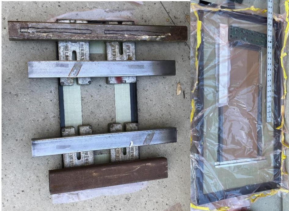
Figure 24: (left) Weighed down composite angles while epoxying. (right) Last J-channel being epoxyed in the upper left corner with protective plastic over to prevent anything from getting on the glass during the cure time.
