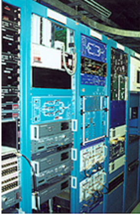
Master Control Station, Montreal Teleport
