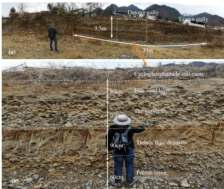
Figure 11. Overview of the artificially excavated slope profile for a house construction near highways
