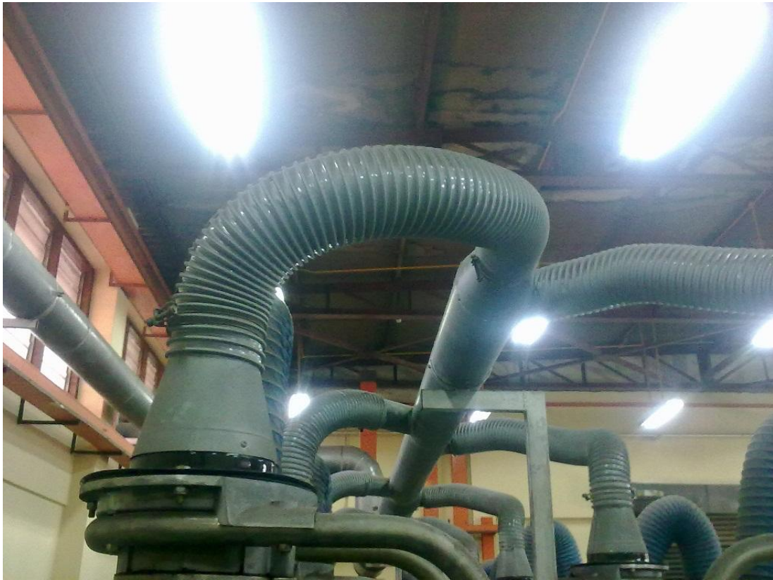
Figure 2.4: An example of ducts at Welding Laboratory in UTHM
