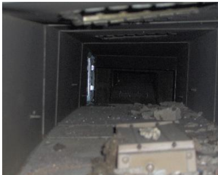
Figure 2.1: Dirty Ducts. Source: http://www.dustbusters.net
