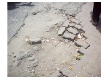
Figure 58. Damaged paving. The few public spaces that exist in DSM are often of poor quality.
