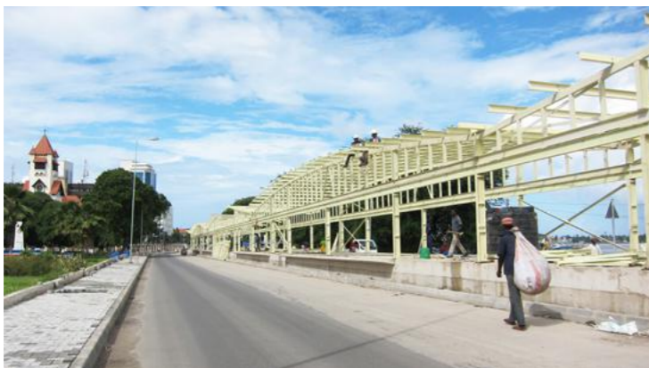
Figure 94. A new bus stop is being constructed in adherence to Bustani ya Posta.
