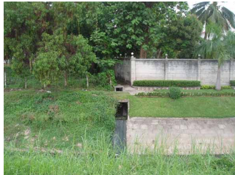
The difference in appearance between public participation and no maintenance at all.
