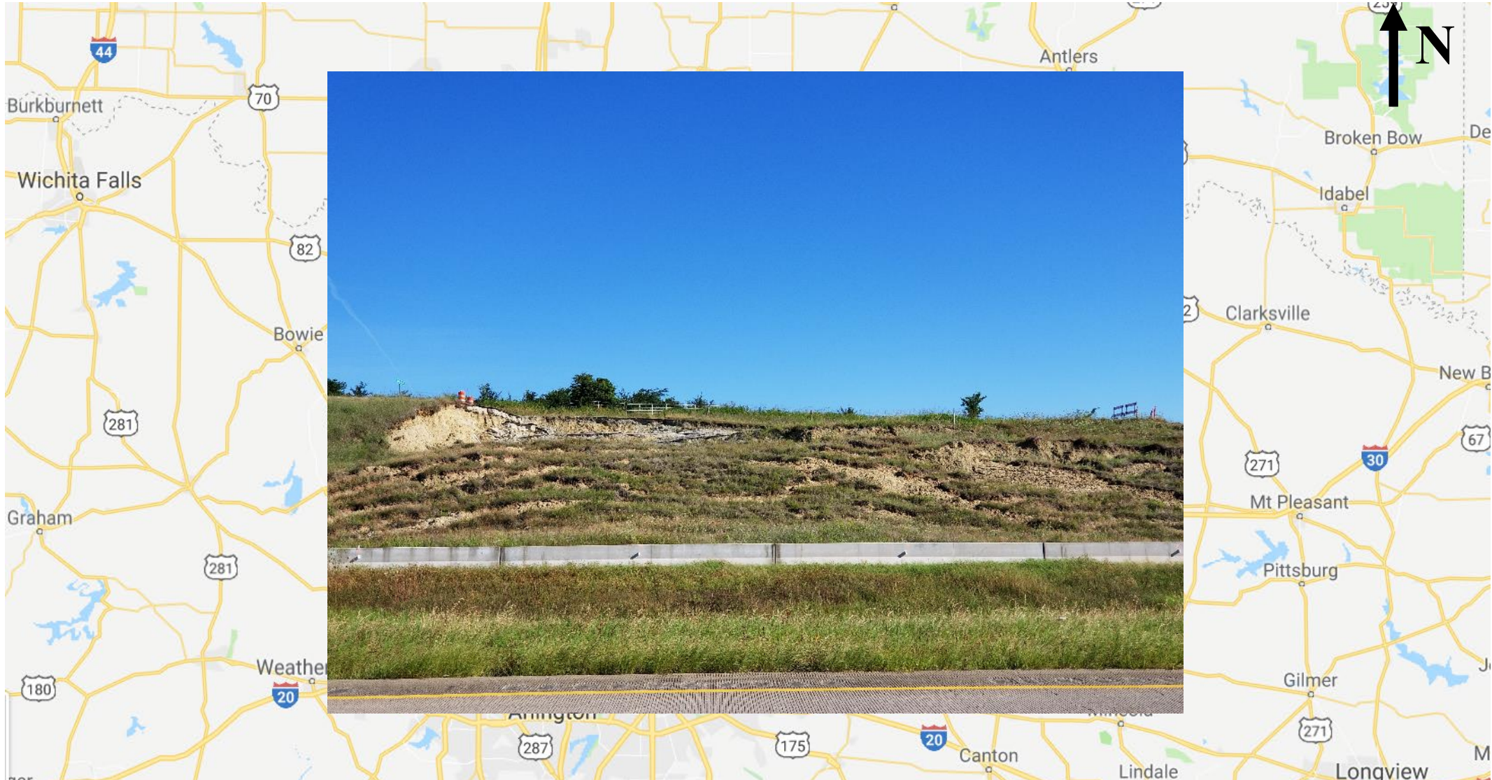
Highway Embankment Slope Failure Along US75: Texas DOT – Paris District
