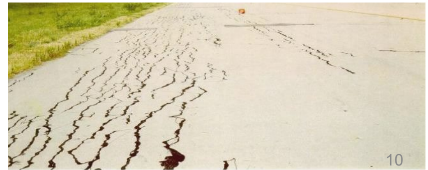
Subsoils Near DFW Airport Sulfate Contents > 30,000 ppm
