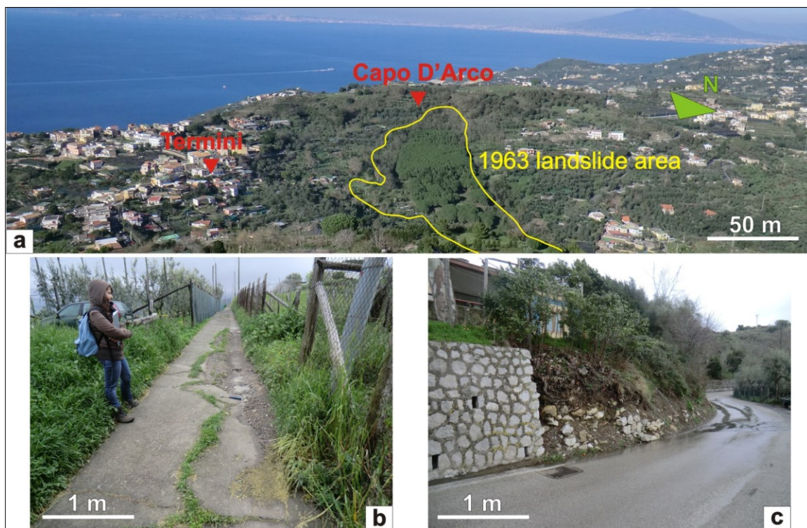
Figure 4.1 – Panoramic sketch of the 1963 landslide's crown area (a). A damaged pathway at Capo d'Arco (b) and a partial collapse of a retaining wall on the provincial road n.192 (SP192; c).
