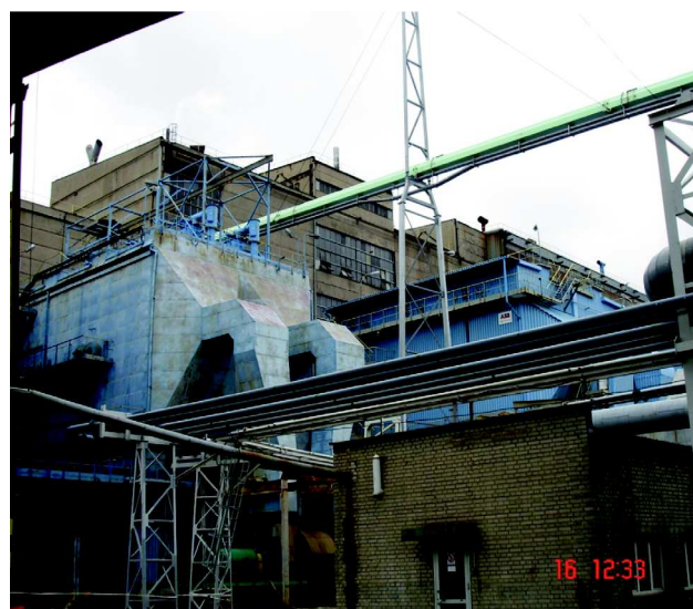
Figure 3. Power block fed with biomass
